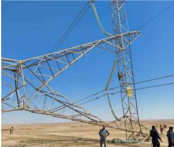
Figure (2): Some of the towers subjected to sabotage
