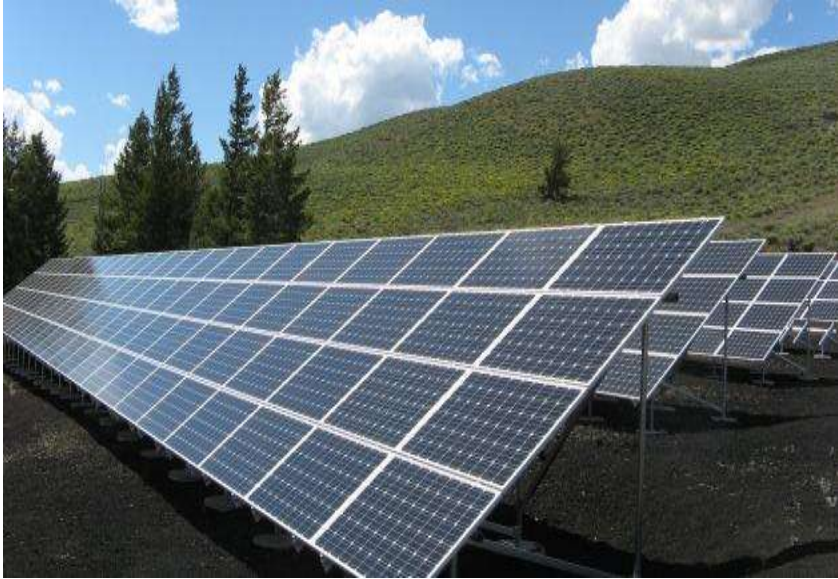
Figure (6): Solar Panels for Electricity Generation
